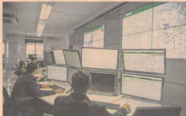
Network operation center
